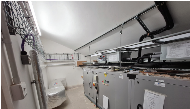
HEPA airfiltration units installed at the new quarantine laboratory
